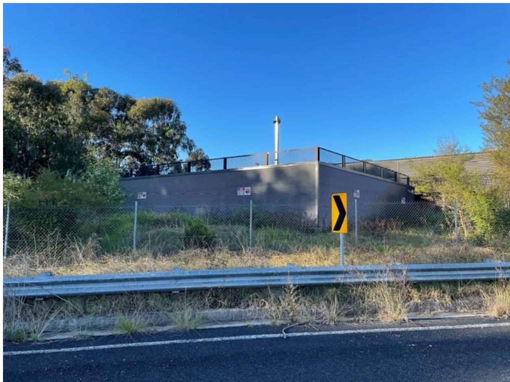
Phot 2. Sydney Trains HV substation located approx. 66m from the property fence.
